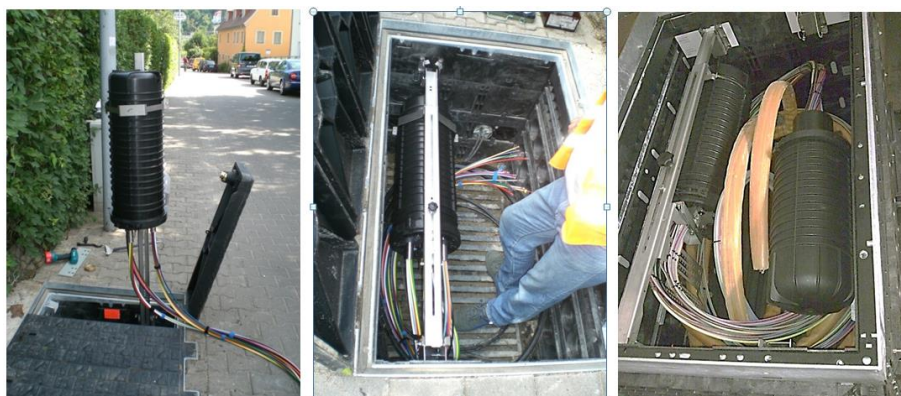
Figure 13: Underground fibre distribution with closures
